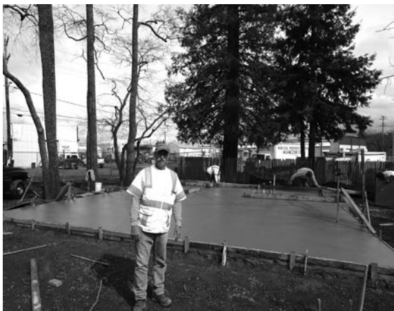
Rick Cupples, of Cupples Construction, in front of the newly poured foundation for the Outdoor Classroom.
